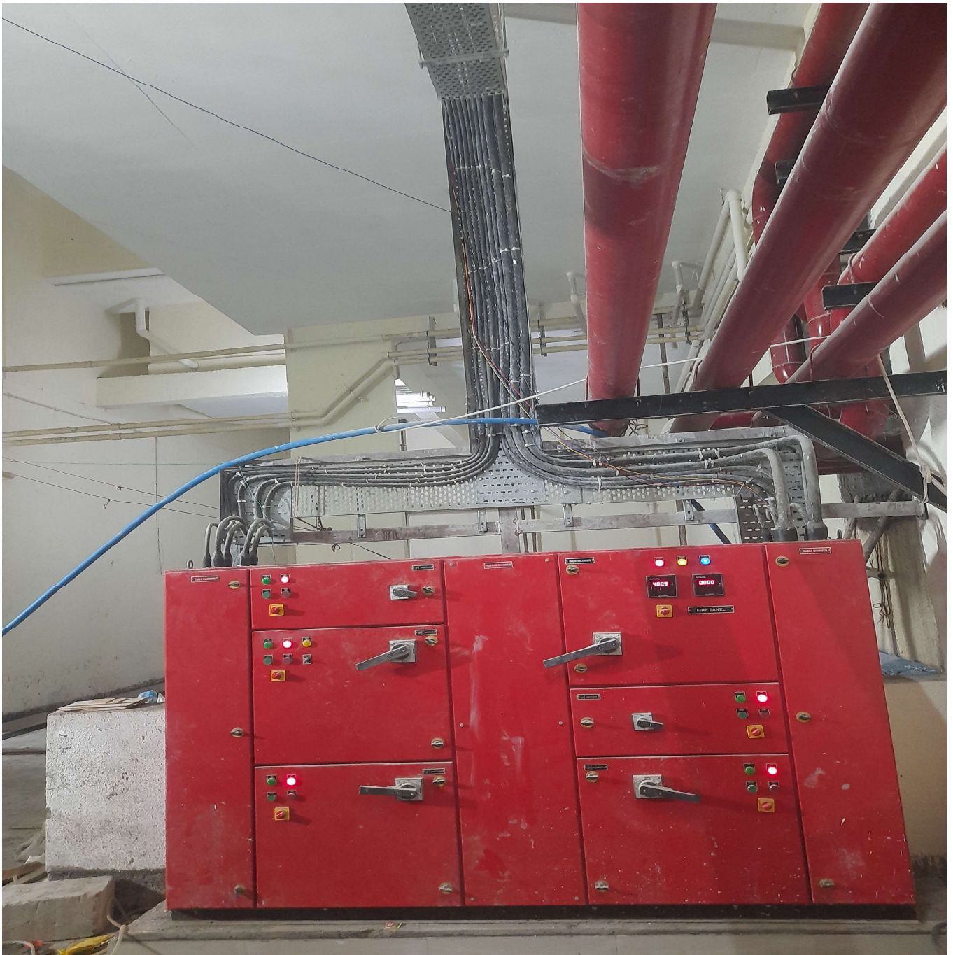
Al-Jamea Fire Panel Cable Termination
